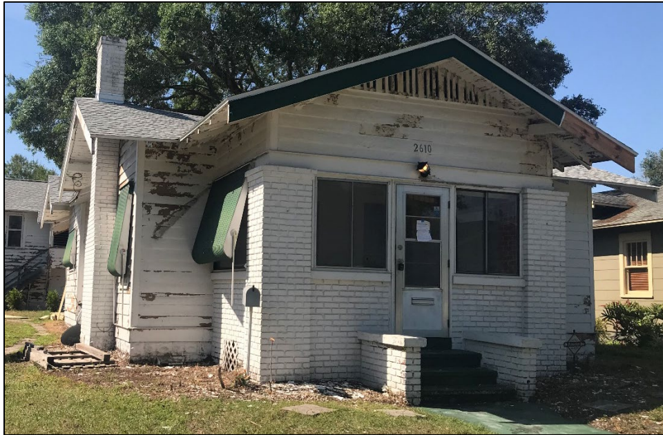
Figure 2: Photograph of house submitted by applicant, prior to unpermitted work.
