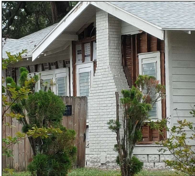
Figure 1: Photograph submitted to the Urban Planning and Historic Preservation Division, showing significant siding removal without a building permit or a Certificate of Appropriateness.
